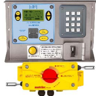
Amplifier conveyor station complete with telephone keypad, pullswitch, interrogate button, and remote isolation
